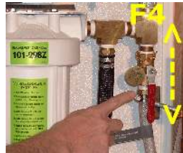
Open Filter Flush to Drain Valve F4 to relieve pressure.
