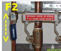
Open Filter Flush Valve F2 (handle parallel to pipe).
