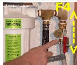
Flush filters using Flush to Drain Valve F4. 4 minute flush required.
